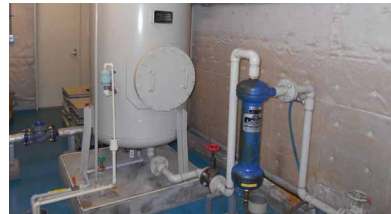
IIF Mitaka Card Center Automatic water supply apparatus
